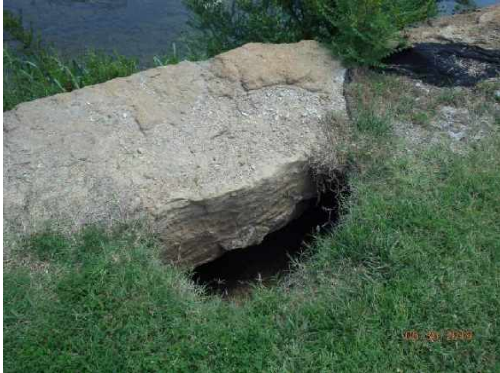
B – HOLE REPAIR - $500
