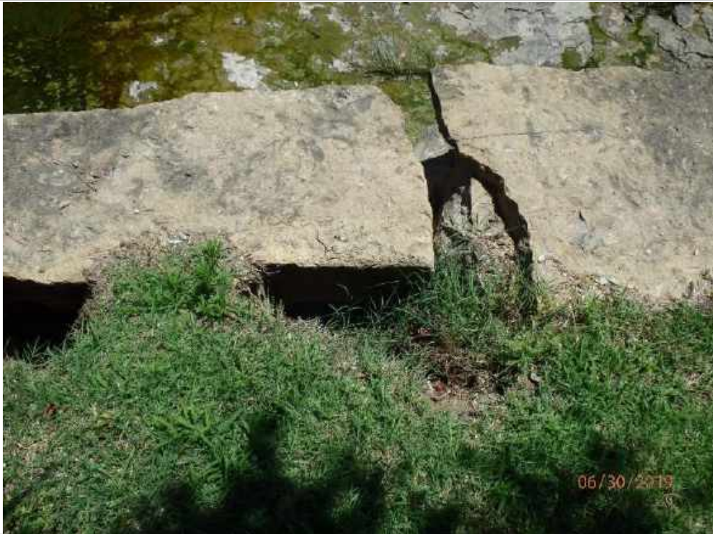
D – HOLE REPAIR - $500
